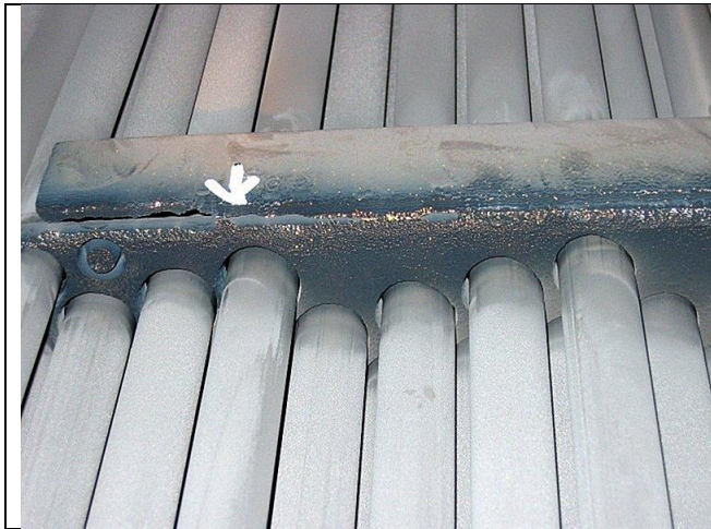
Figure 7 – Erosion of Tubes and Side Bars in a vertical FWH
