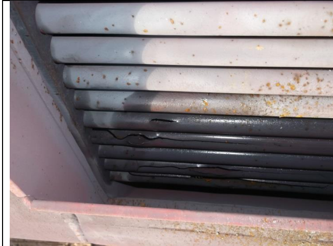
Figure 5 – Failures at the DC Entrance window due to low liquid level
