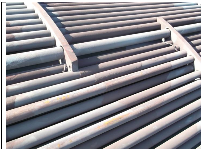
Figure 1 – Areas of two-Phase flow can be seen near DC Zone Baffels
