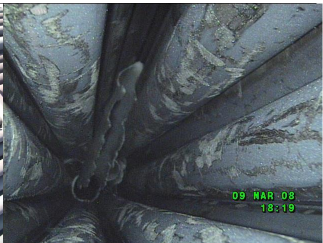
Figure 2 – Tube Damage due to flashing within a Drain Cooler Zone
