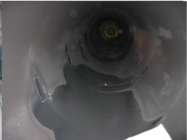
Figure 8 – Flow accelerated corrosion of Vertical FWH Shell due to moisture entrained in the steam.
